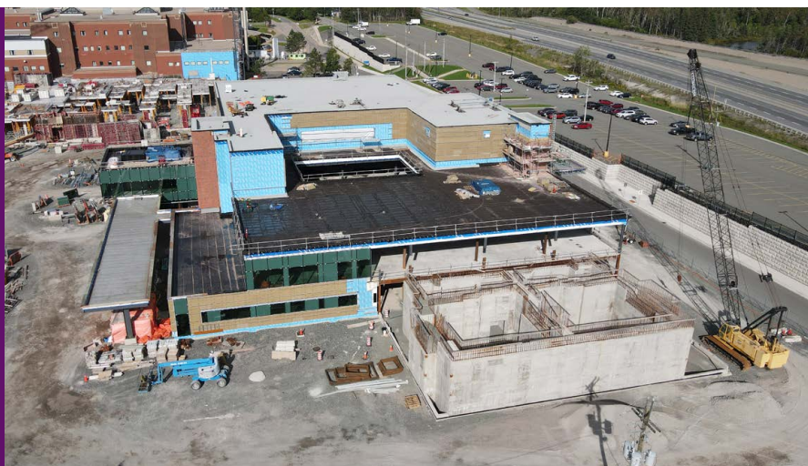
Pictured here is the progress made on the construction of Cape Breton's new Cancer Centre as of September 2023
